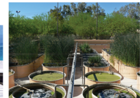
Living Machine with cisterns
